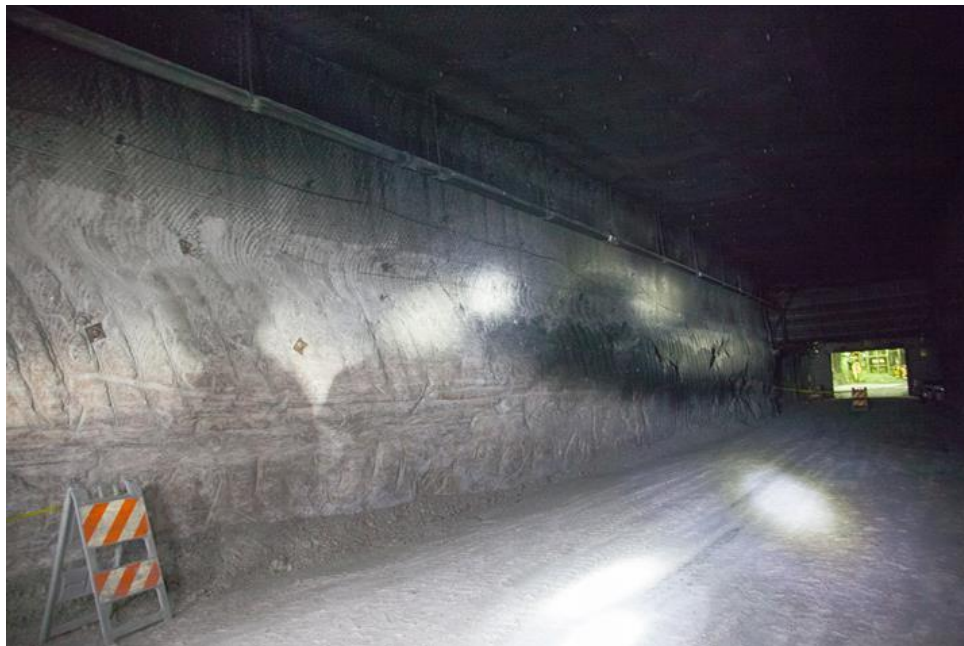
Figure 23: Smoke Signature on Rib (Looking South)
