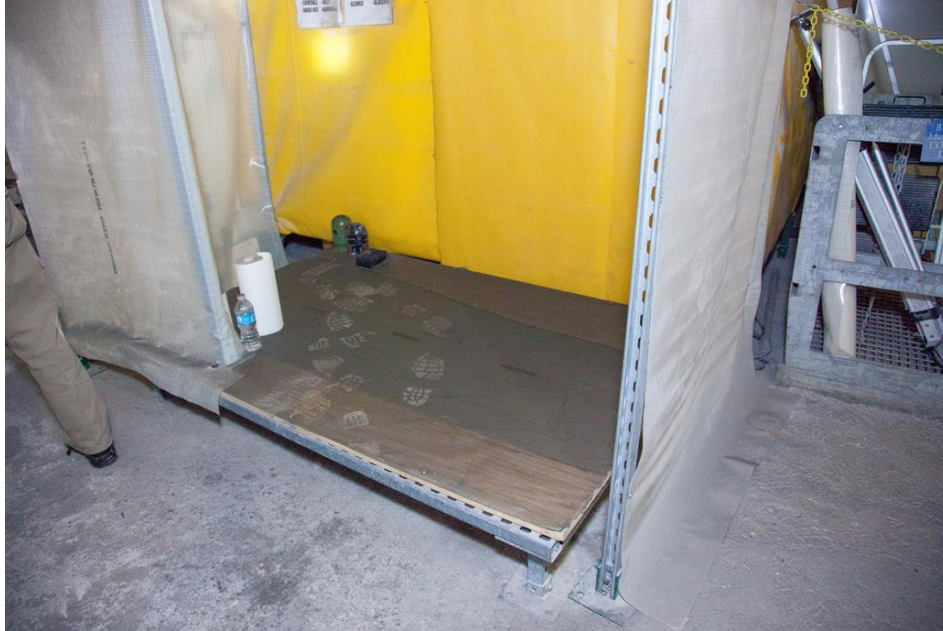
Figure 24: Soot Deposits in North Ventilation Circuit
