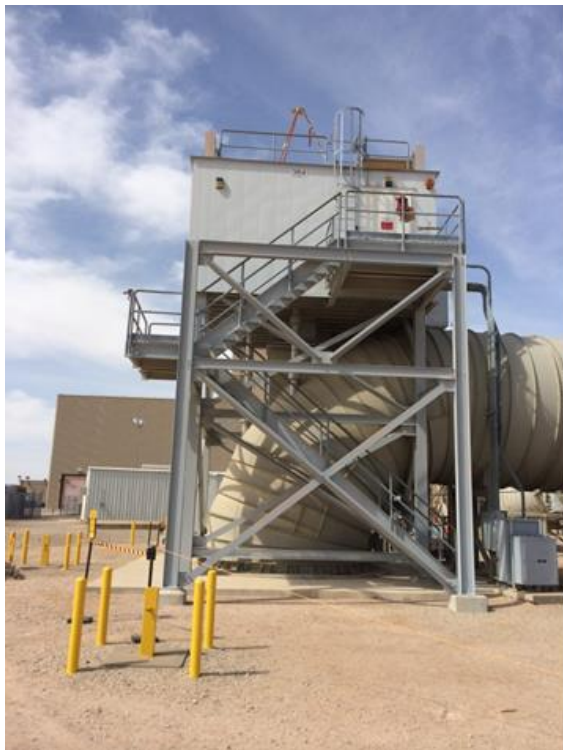
Figure 8: Ventilation Sample Station A
