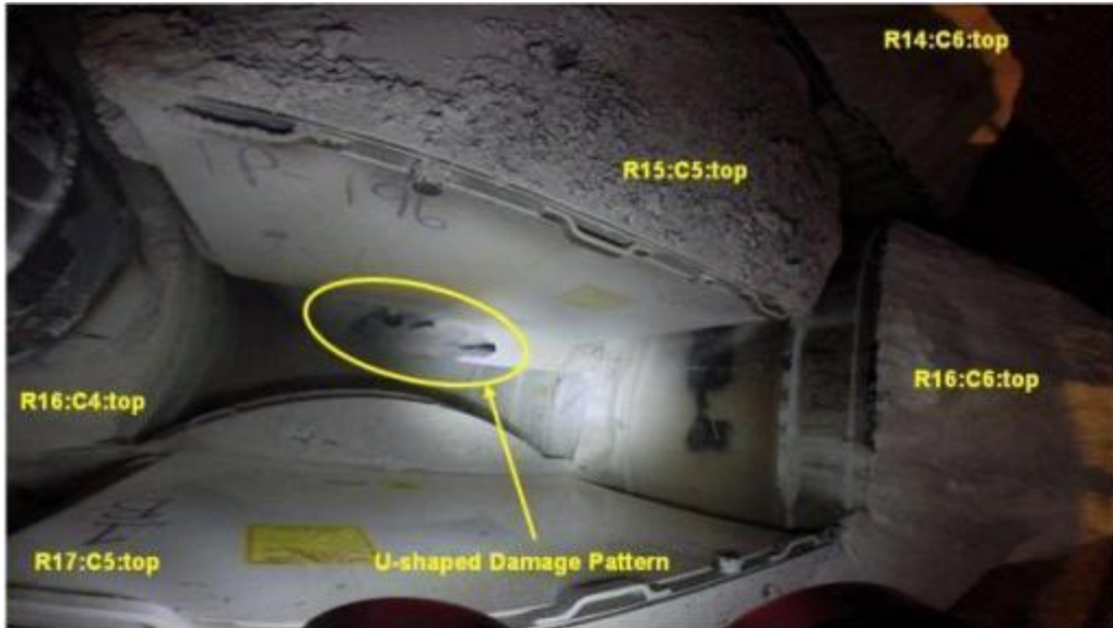
Figure 6-37: Damage to Slip Sheet at R15:C5
