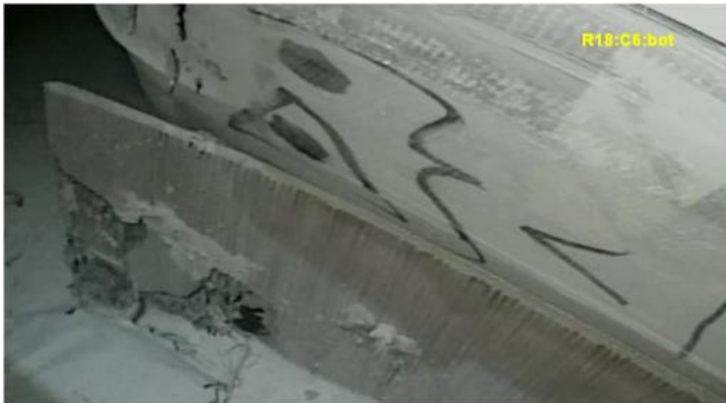
Figure 6-16: Face View (west) – Debris at Base of R18:C6
