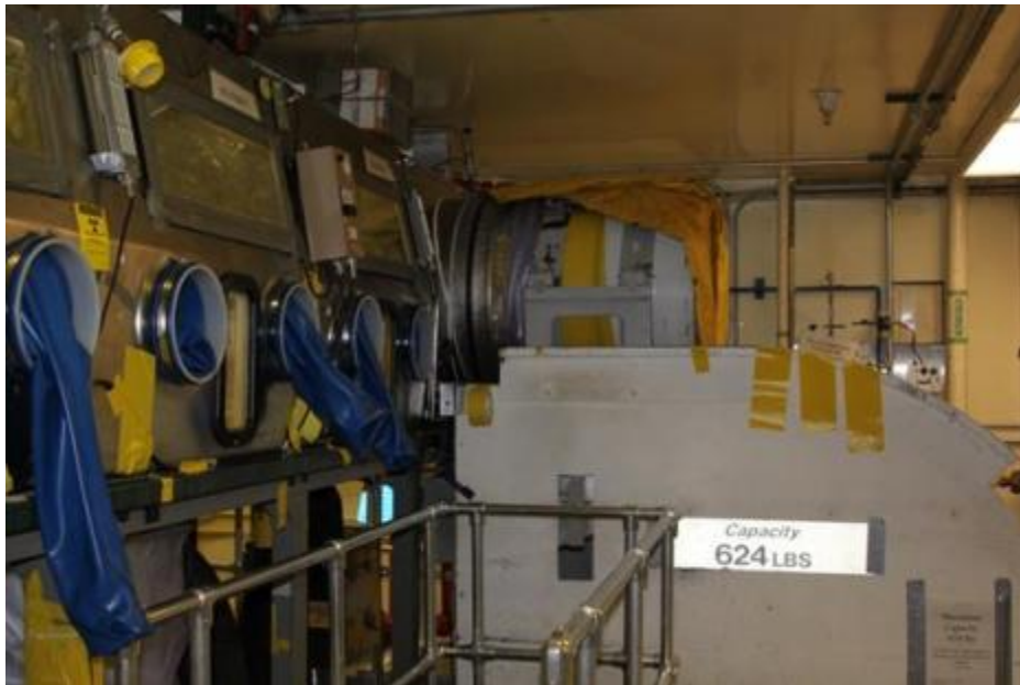
Figure 1-7: Waste Characterization Glovebox in WCRRF at LANL
