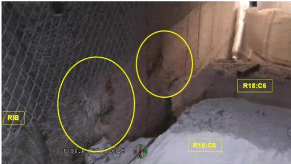
Figure 6-17: Rib Damage near Rows 16 and 18
