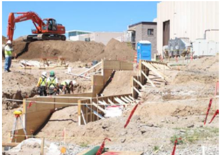
Construction of Radioactive Liquid Waste Treatment Facility (RLWTF), Technical Area 50. LANL Project Overview and Status presentation, April 18, 2016. ( LA-UR-16-23398 )
