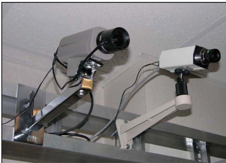
Figure 13-6. Physical Security Systems provide security technologies deployed throughout NNSA sites.
