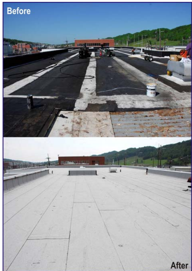
Figure 11-2. Roof repairs on Building 9113 at Y-12. FIRP replace 21,300 square feet of roofing on time and within budget.
