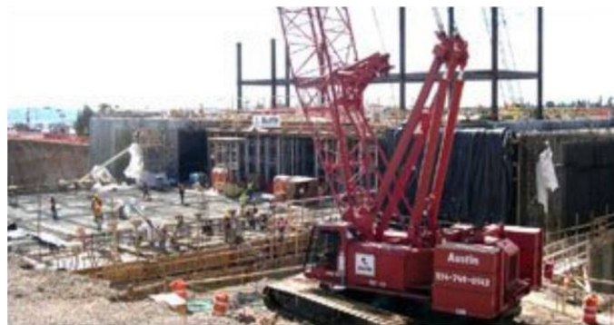
Figure 1-12. The Radiological Laboratory Utility Office Building at LANL is scheduled for completion in 2009.
