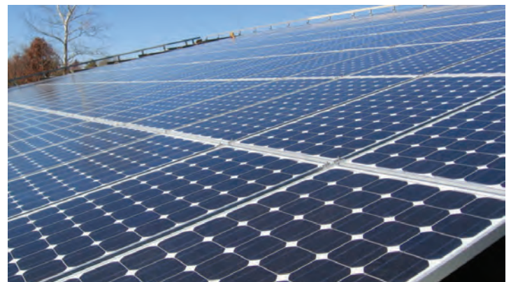
A 3-megawatt fixed-tilt solar photovoltaic array is scheduled to be built on 10-acres in the northwest buffer zone through a power purchase agreement. The facility is expected to generate approximately 6,300 megawatt-hours annually. This system will represent the DOE/NNSA’s largest purchase of solar power from an onsite facility and the first in the western region.
