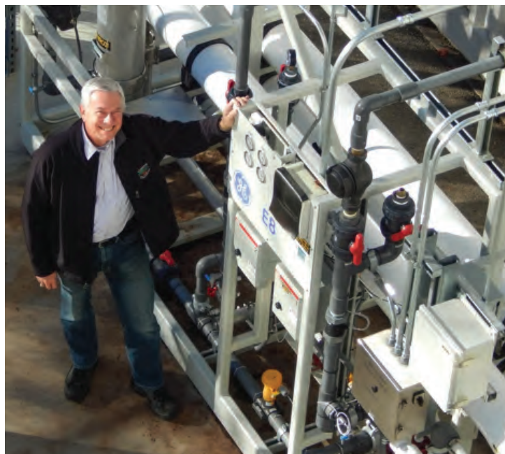
Being sensitive to California’s current drought conditions, this reverse osmosis unit recycles water for a cooling tower—one of the sustainability measures that has allowed the Laboratory to save more than 10% of the water it consumes annually.
