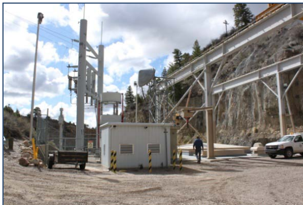
Figure 3: El Vado Electric Power Plant
