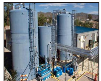
Sanitary Effluent Reclamation Facility
