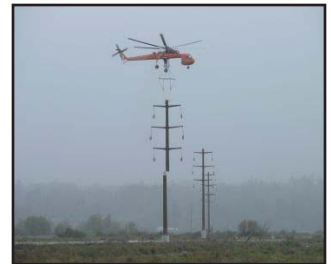
Additional 115kV Transmission Line
