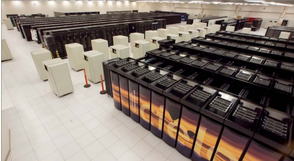
Figure 21. SCC Data Center Showing Cielo the Proposed Trinity Location
