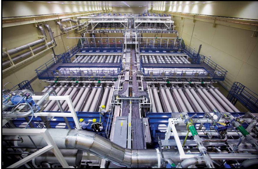
Figure A-5-3. One of two identical NIF laser bays, viewed from above. Each laser bay has two clusters of 48 beamlines.
