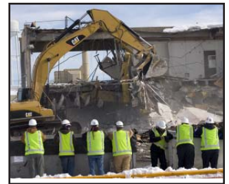
D&D of TA-21 (DP East, West, and the Tritium Systems Test Assembly Facility)
