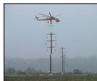
Additional 115kV Transmission Line
