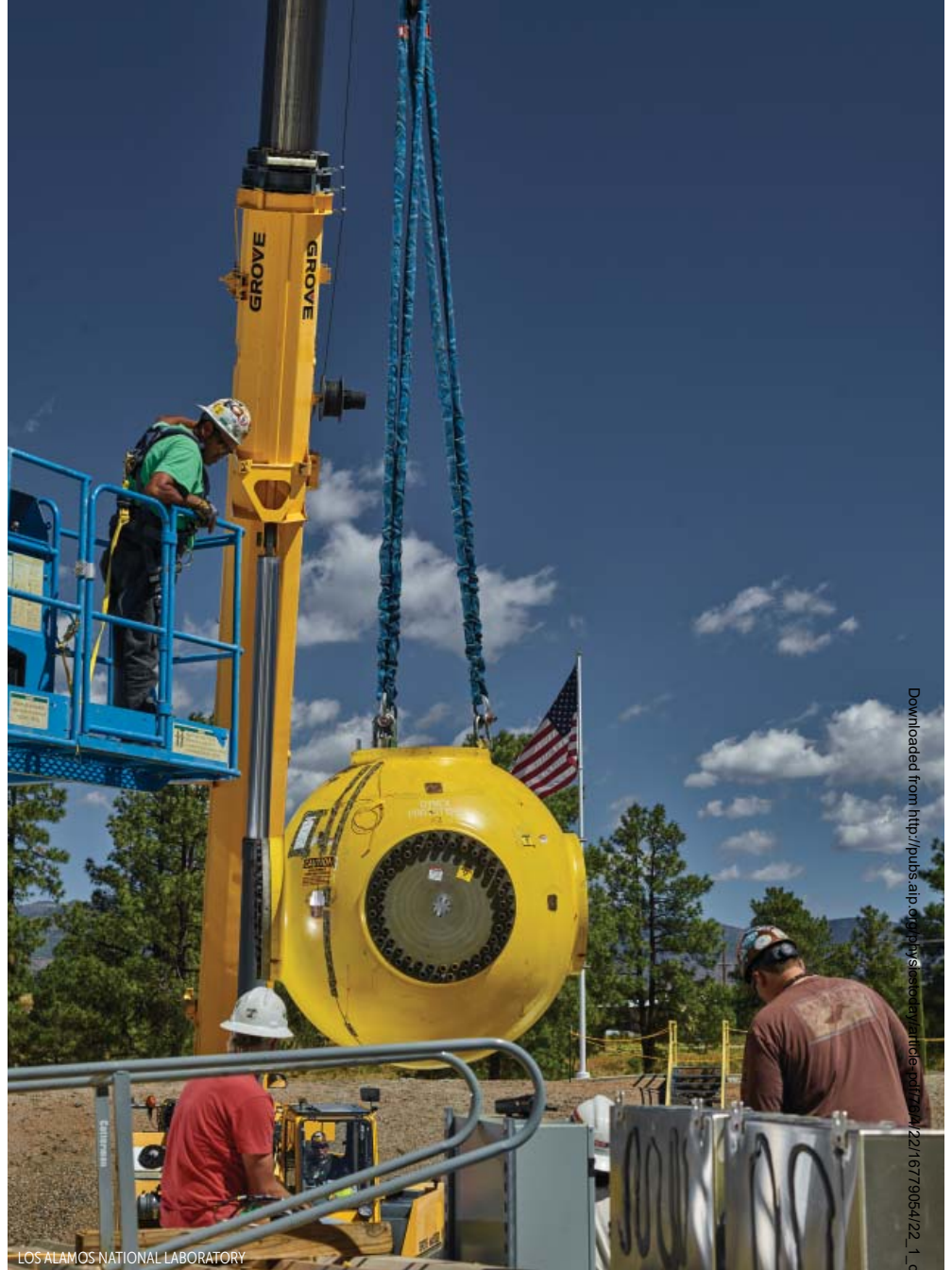
A BLAST CONTAINMENT chamber is lowered into place at the Dual-Axis Radiographic Hydrodynamic Test facility at Los Alamos National Laboratory. Explosive tests on mock pits made from surrogate metals are used to help determine how plutonium will compress as the pit of a nuclear weapon implodes.
