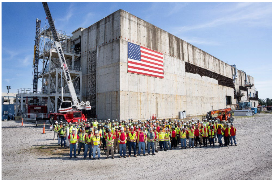
SRNS subcontractor Aecon-Wachs performed the dismantlement and removal (D&R) of equipment and commodities from the Savannah River Plutonium Processing Facility (SRPPF) at the Savannah River Site (SRS).
