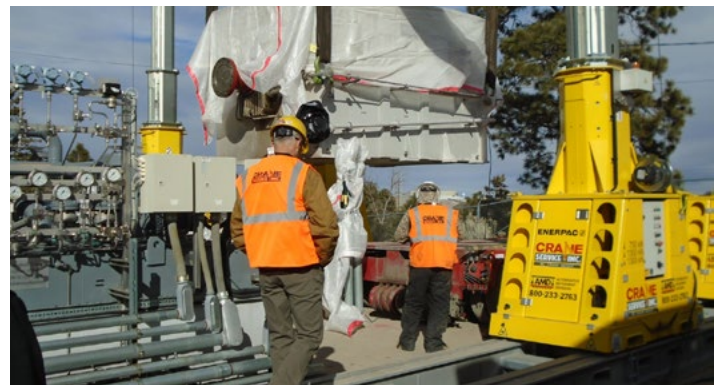
Subcontractors install the new combustion gas turbine generator at the TA-03 steam plant.
