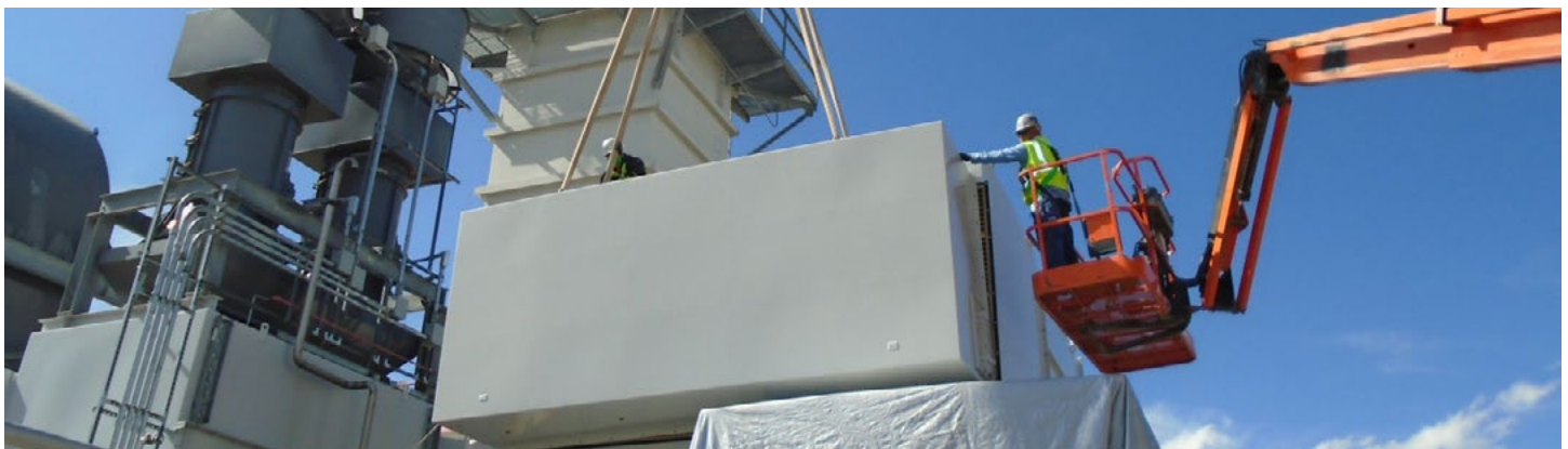
The new combustion gas turbine generator was installed in April 2020 and conditionally accepted by the NNSA in September.
