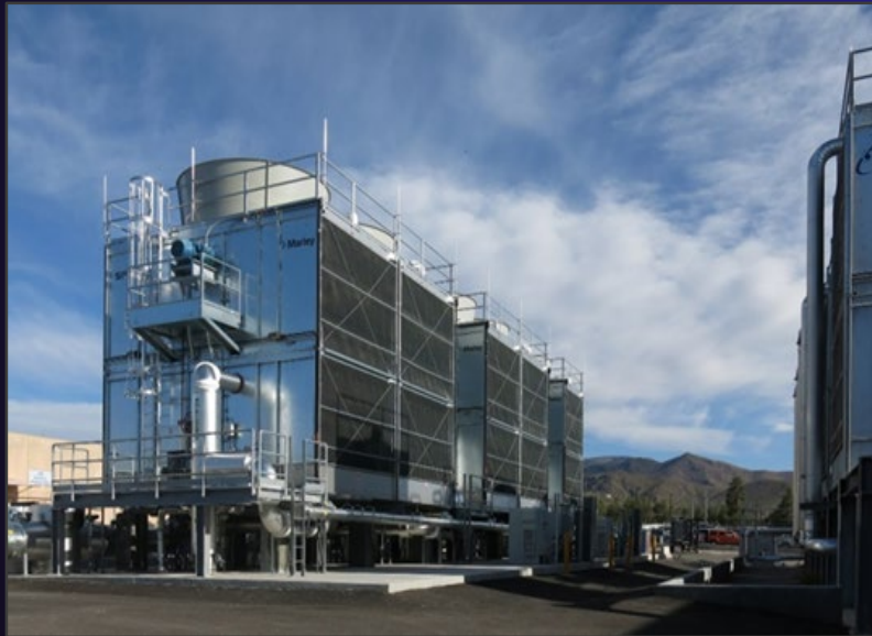
Exascale Class Computer Cooling Equipment Project
