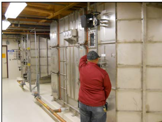
Figure 6. Air Filters in RLUOB
