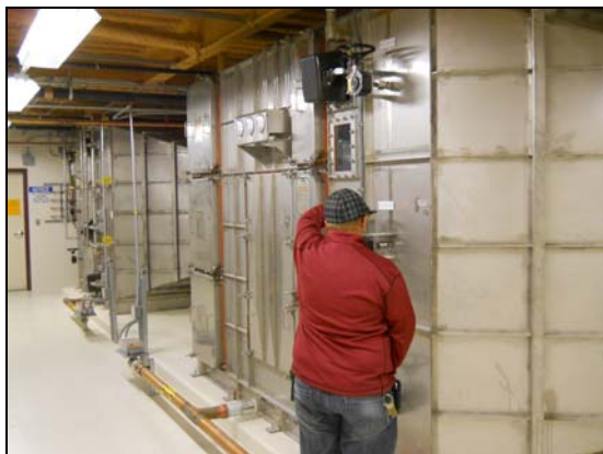
Figure 6. Air Filters in RLUOB
