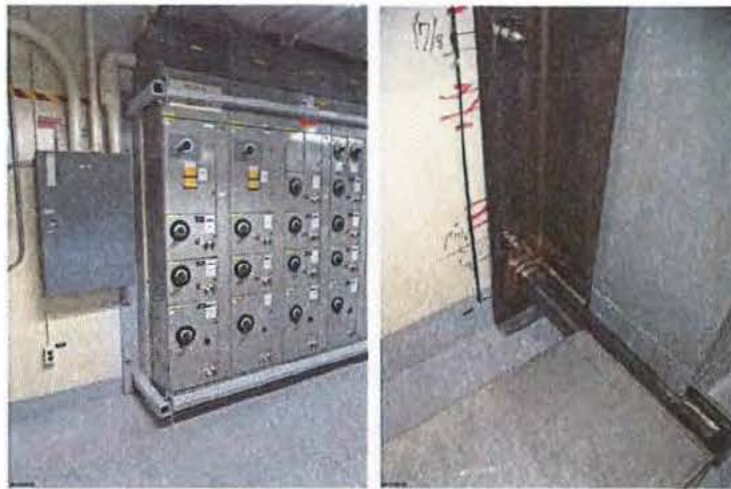
Figure 6. Motor Control System Anchorage
