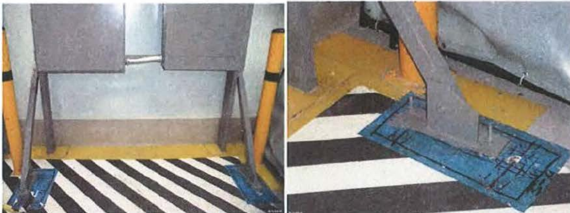
Figure 7. Anchorage of Uninterruptible Power Supply Auto Transfer Switch
